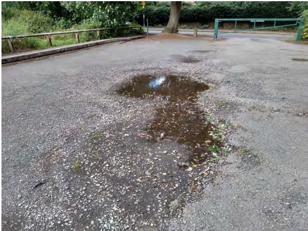
Puddling in Parking Area
